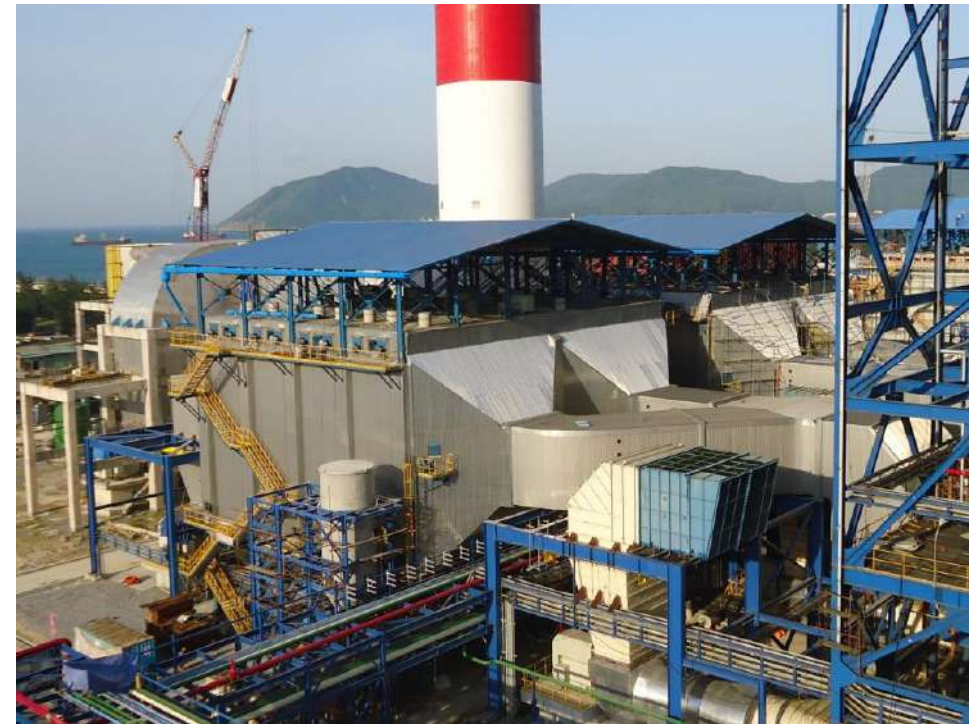
ESP after thermal insulation
